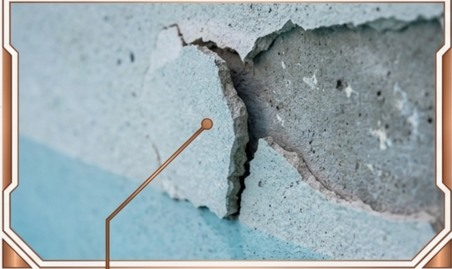
Chipping & Peeling | STRUCTURAL FAILURE
